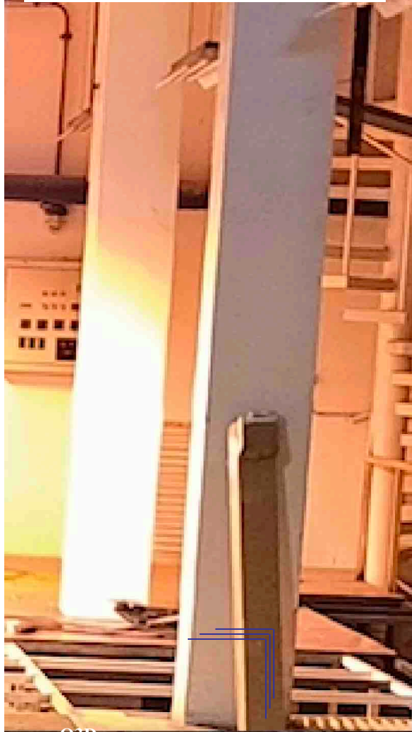
Post Accelerator basement
